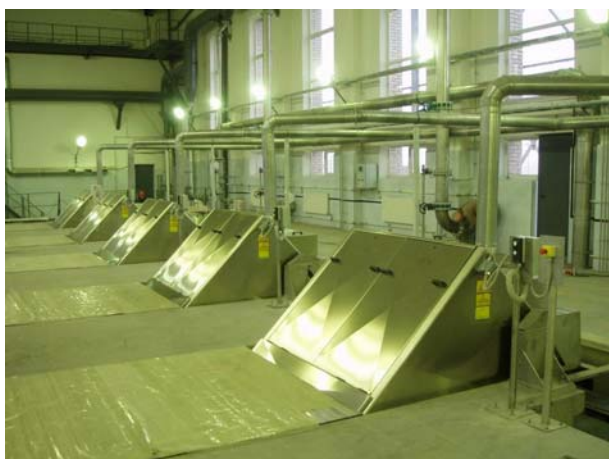
(Above: New grit removal station at the Northern Incinerator project in St Petersburg) Photo courtesy of Rambøll Danmark A/S
