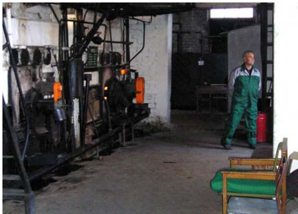
(Above: inside a boiler house in Kaliningrad)
