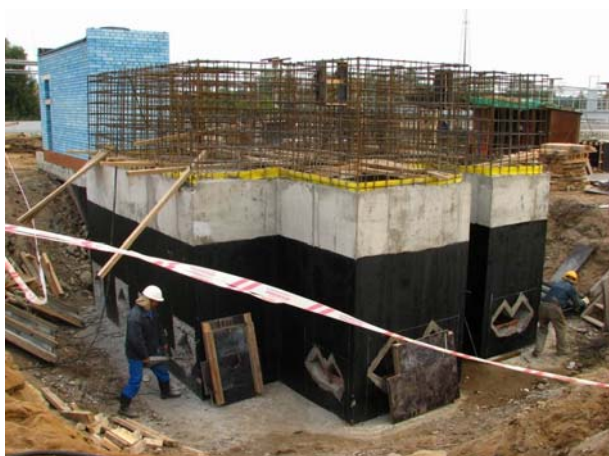
(Above: St Petersburg Northern Incinerator project - concrete works at pumping station in November 2006 funded by NDEP grant) Photo courtesy of Rambøll Danmark A/S
