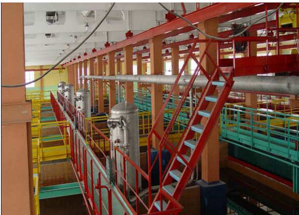
(Above) New water treatment facilities in Block No 4 in Syktyvkar Vodokanal
