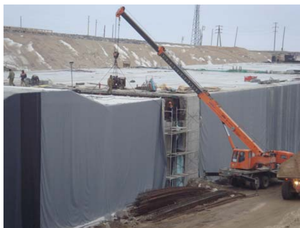
Construction of the underwater tunnel which will lead vehicle traffic underneath the main navigation channel (photo courtesy of Boskalis International BV)
