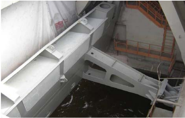
One of the gates inside a water sluice in a raised position (photo courtesy of Jacobs and HR Wallingford)
