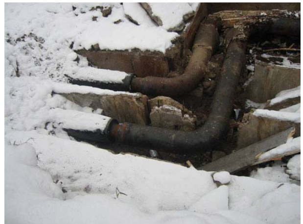
Murmansk district heating system is in dire need of an upgrade
