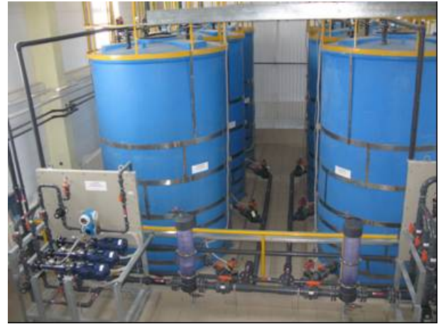
NDEP funded water disinfection system – hypochlorite production station in Syktyvkar
