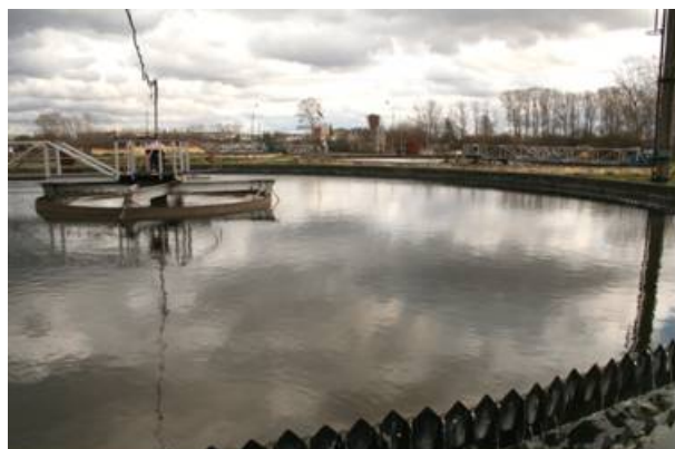
One of the six primary sedimentation tanks at Vologda Wastewater Treatment plant
