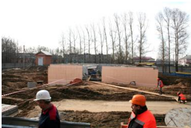
Construction of the aeration and UV-disinfection building at the Vologda Water Treatment plant – funded by EBRD loan
