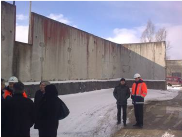
Kaliningrad Wastewater Treatment Plant in March 2010 – the civil works on the site have started
