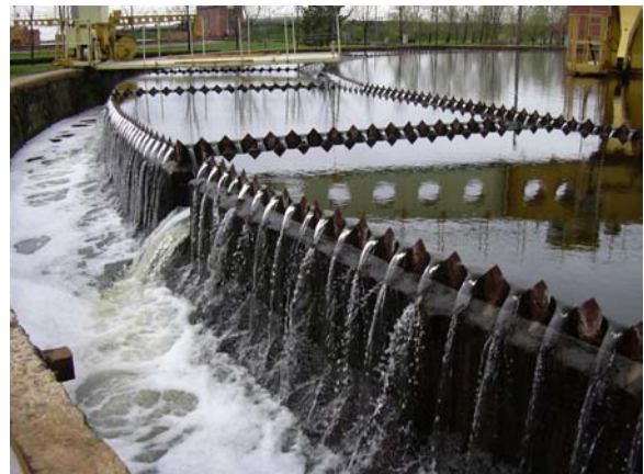
The northern waste-water treatment plant is key to keeping the Baltic Sea waters clean
